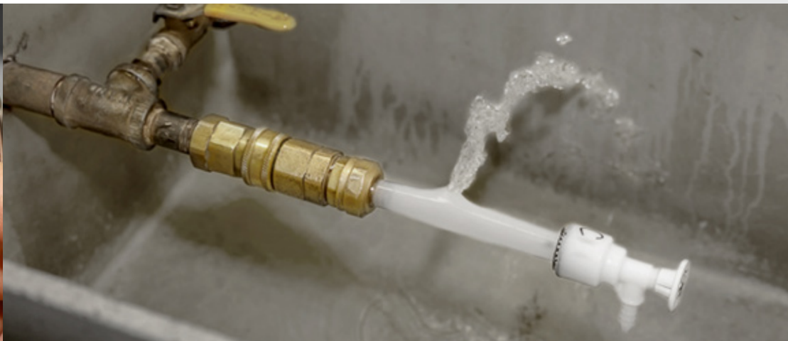
Daily hydrostatic testing. PEX pipe fails during test. ACCOR valve remains attached.
